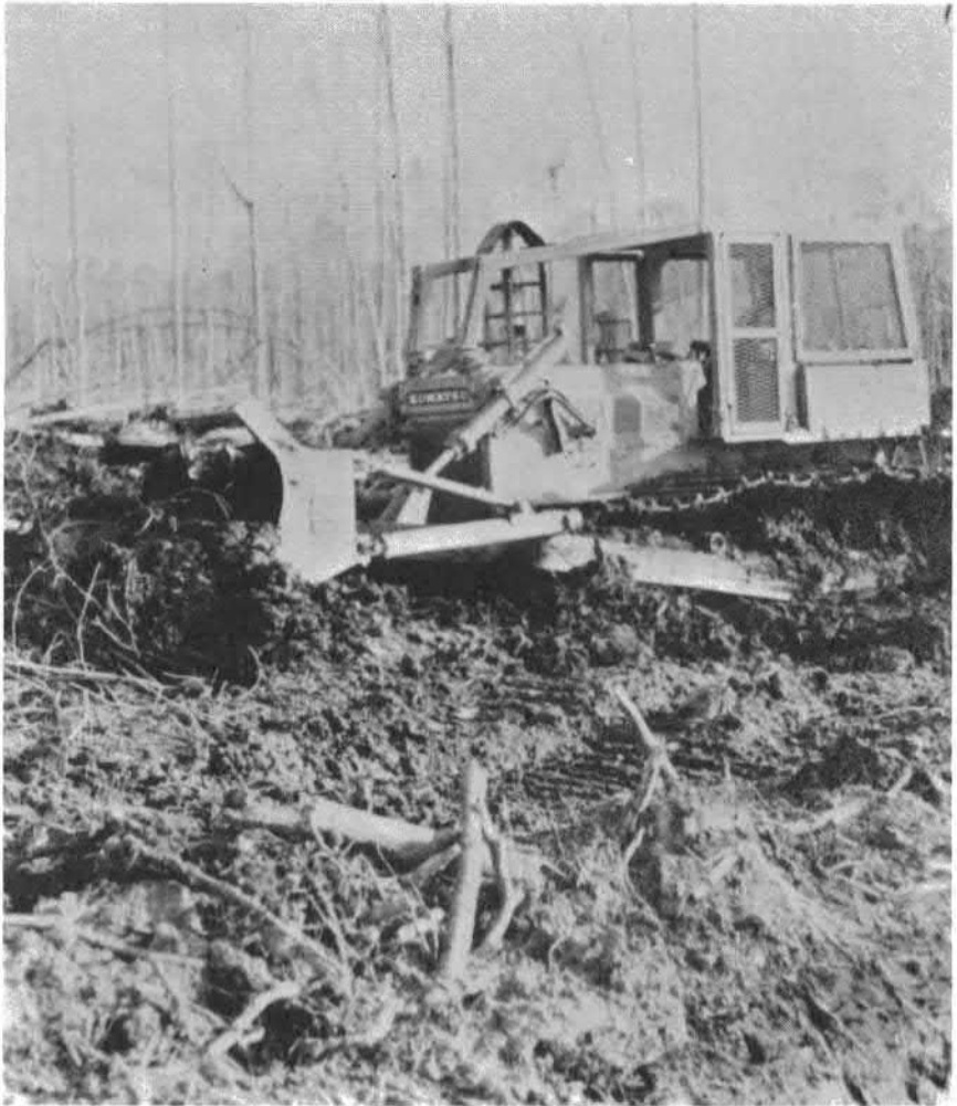
Figure 13. Spoil from the field ditch being moved toward the center of the field during the land clearing process.
