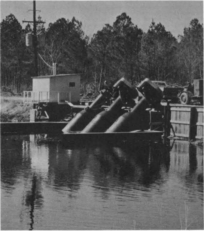
Figure 20. Pumping station with tide gates to remove excess water from low-lying farm land.
