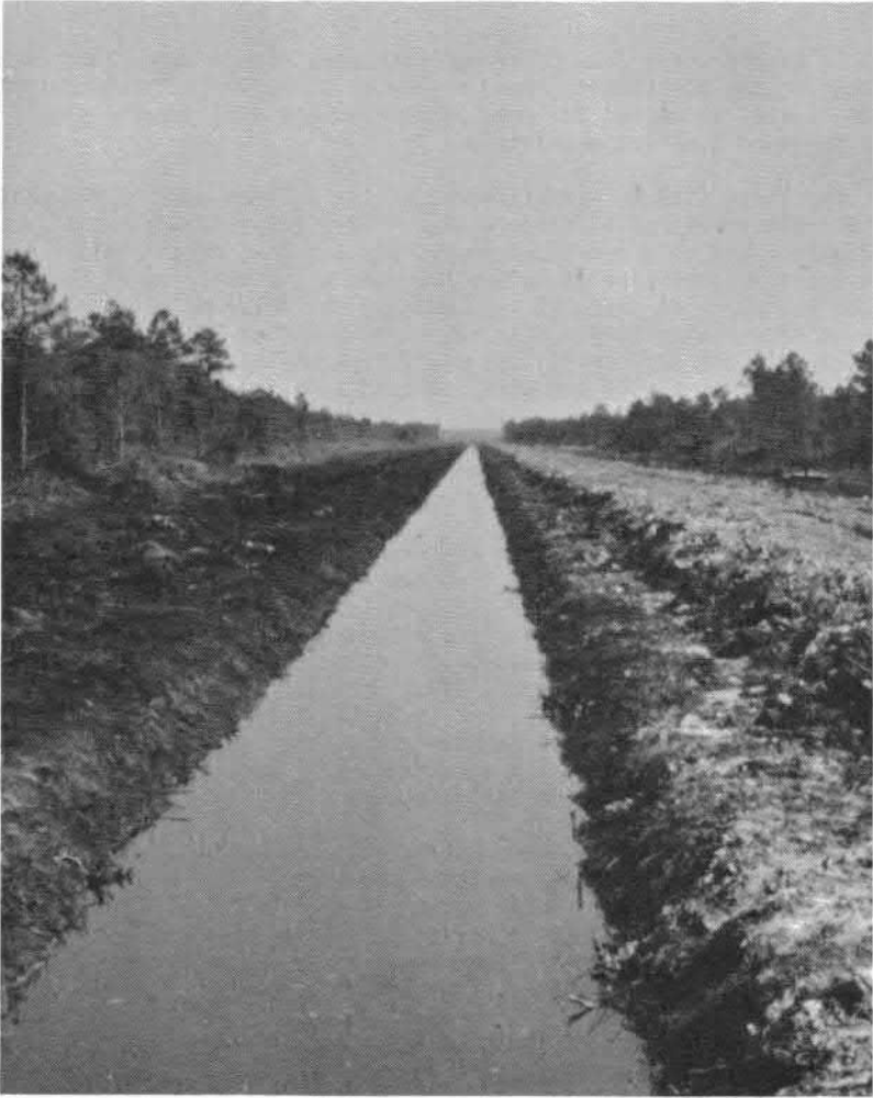
Figure 10. Primary canal system being dug as the first step in land clearing and development.
